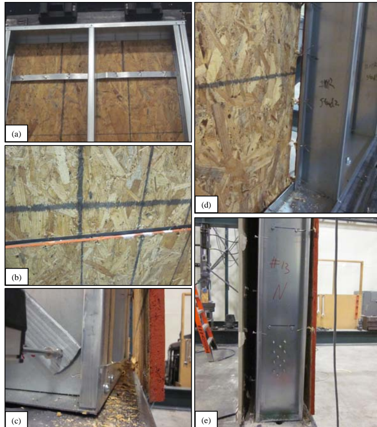
Figure 6 Detailed shear wall response (a) back of test 4, demonstrating fastener pull-through (PT) along the horizontal seam, (b) front of test 2 depicting the resulting separation of sheathing from seam as a result of PT, (c) separation of OSB from bottom of wall track in test 13, (d) Fastener PT and tear-out (TO) against sheathing along field stud in test 11, and (e) north chord stud in test 13, demonstrating fastener PT in the OSB and a combination of PT and bearing (B) in the gypsum.
