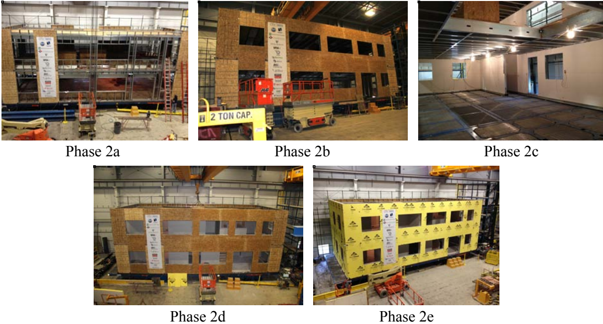
Figure 3. As-built sub-phases of Phase 2 testing. Note, in Phases 2c and 2d, additions are only made to the interior of the building.
